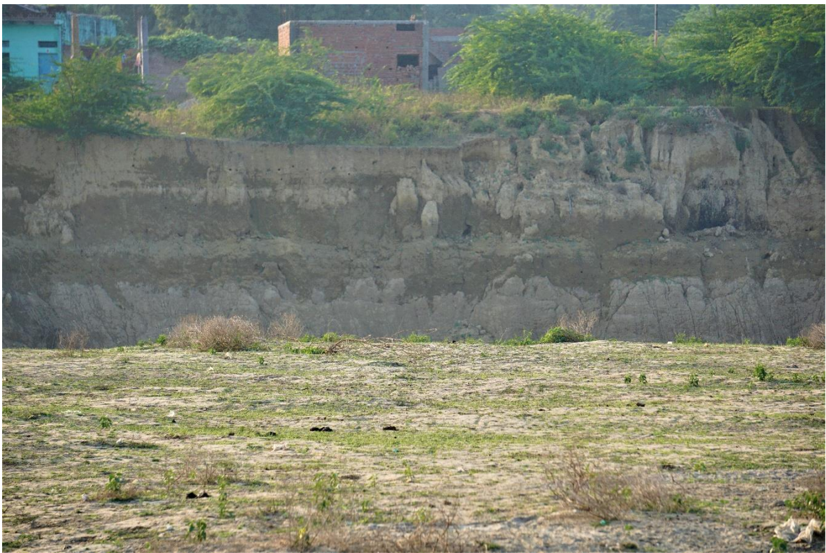
Image 63 : Eroded Bank Of Ojhala Nala Near Ganga-Ojhala Confluence [Left Bank]
