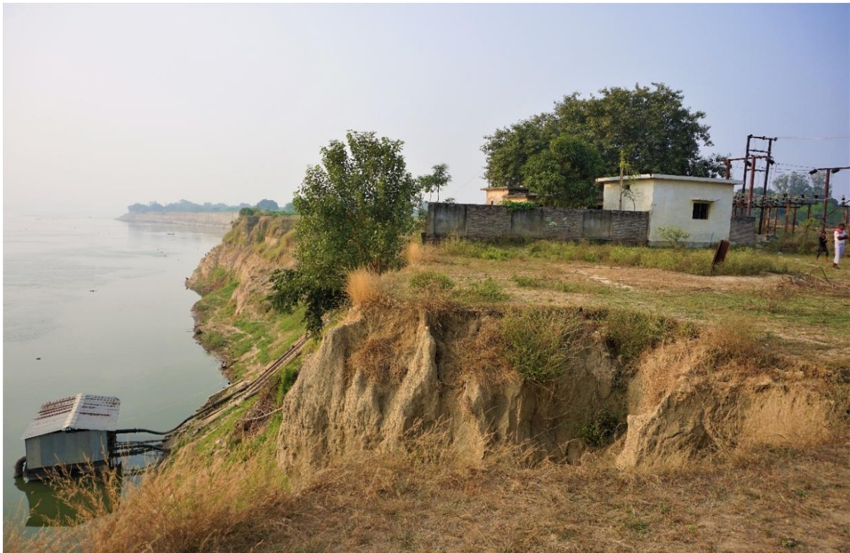
Image 61 : Lateral Erosion Near Hargarh [Right Bank]
